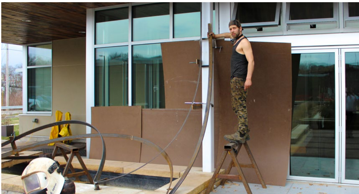
ARTIST INSTALLING WORK AT THE PHIPPS CENTER FOR SUSTAINABLE LANDSCAPES, PHIPPS CONSERVATORY AND BOTANICAL GARDENS.
