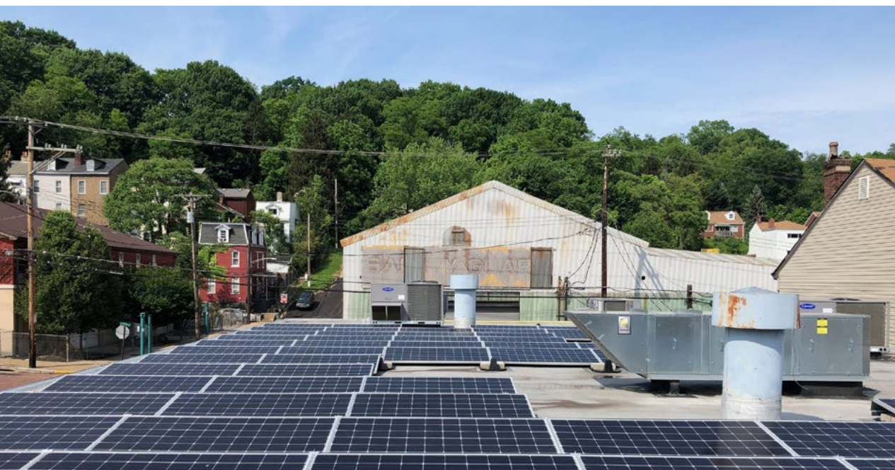
SOLAR ARRAY AT THE MILLVALE FOOD + ENERGY HUB. IMAGE COURTESY OF NSR.
